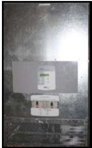
ComEC 160Ampere installed after Mains
