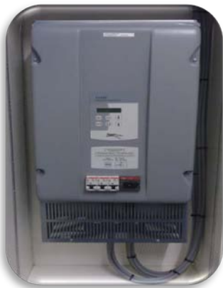
ComEC installed after main switch in electric cabinet
